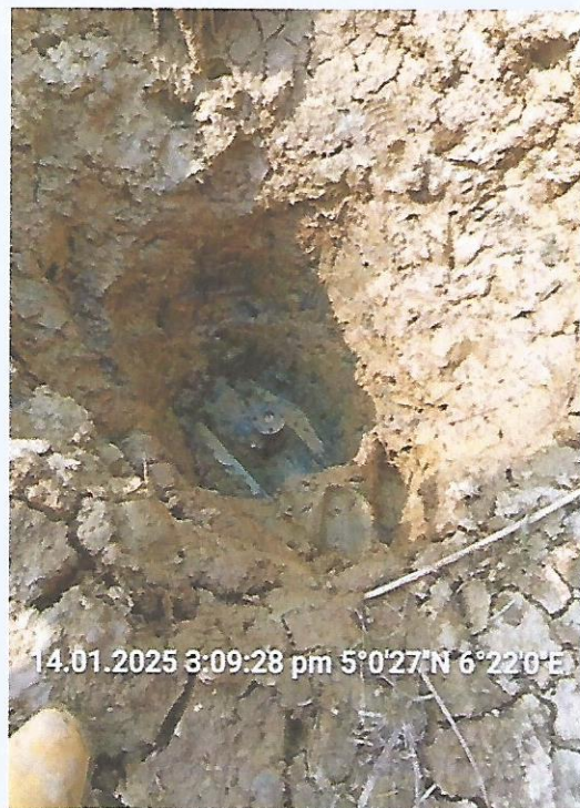
Fig 1: Picture showing the Incident Point.
